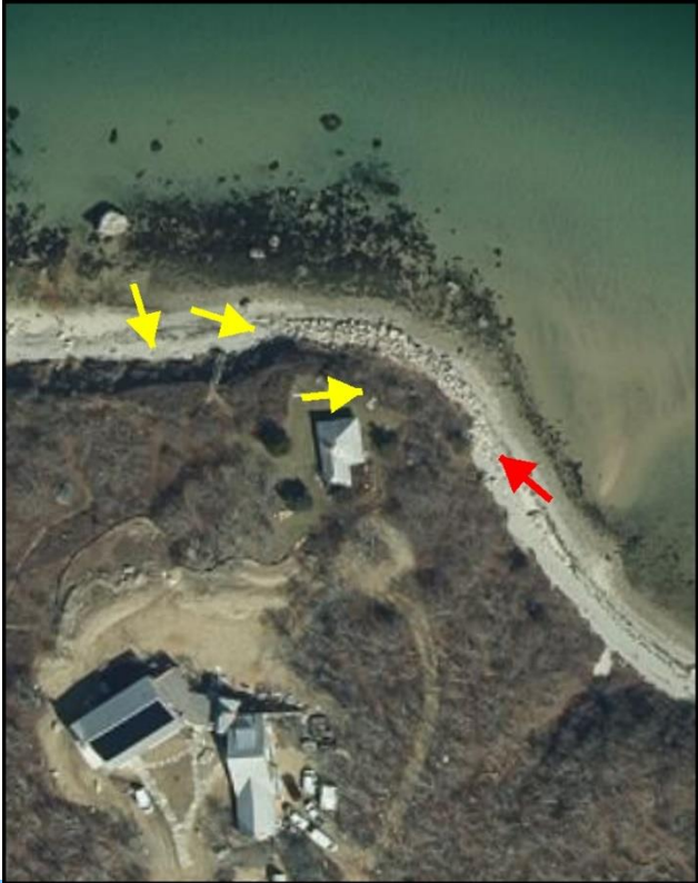
Photograph 2. The eastern end of the existing revetment extends further seaward than the adjacent shoreline. A cobble deposit extends 5-10' from the toe of the coastal bank.
