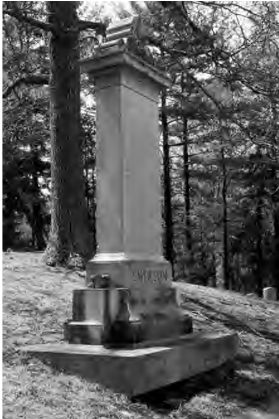
Exposed foundation of Emerson monument
