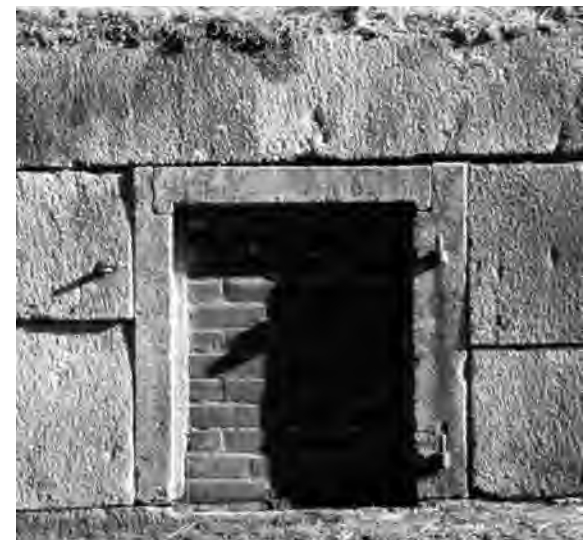
Brick infill at vault entrance, Common Burying Ground, Templeton
