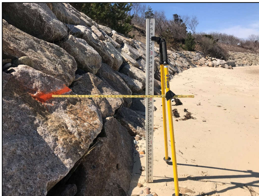
Monitoring Station #2: Beach at elevation 4.9 ft NGVD (2.1 ft below survey mark) on April 14, 2020.
