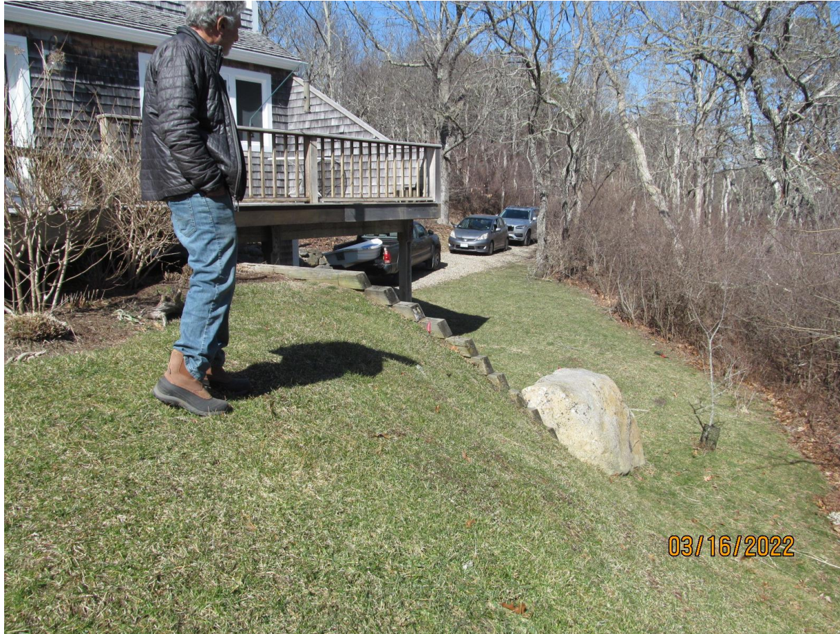
wooden timbers failing and need to be replaced
