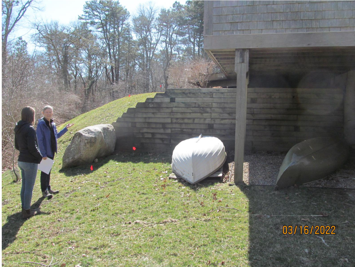
wooden timbers to be replaced with concrete wall.
