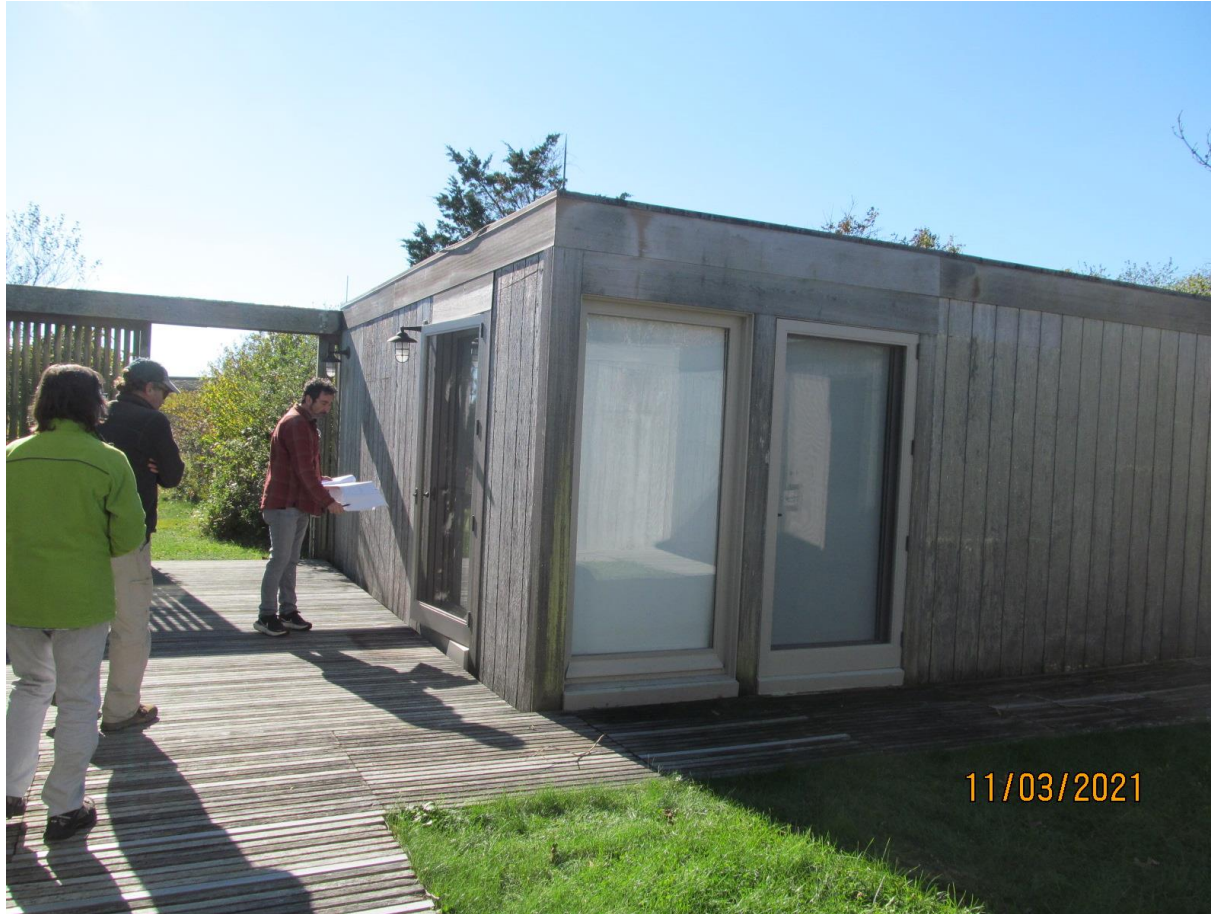
Building 1. To be demolished and rebuilt due to mold problem.
