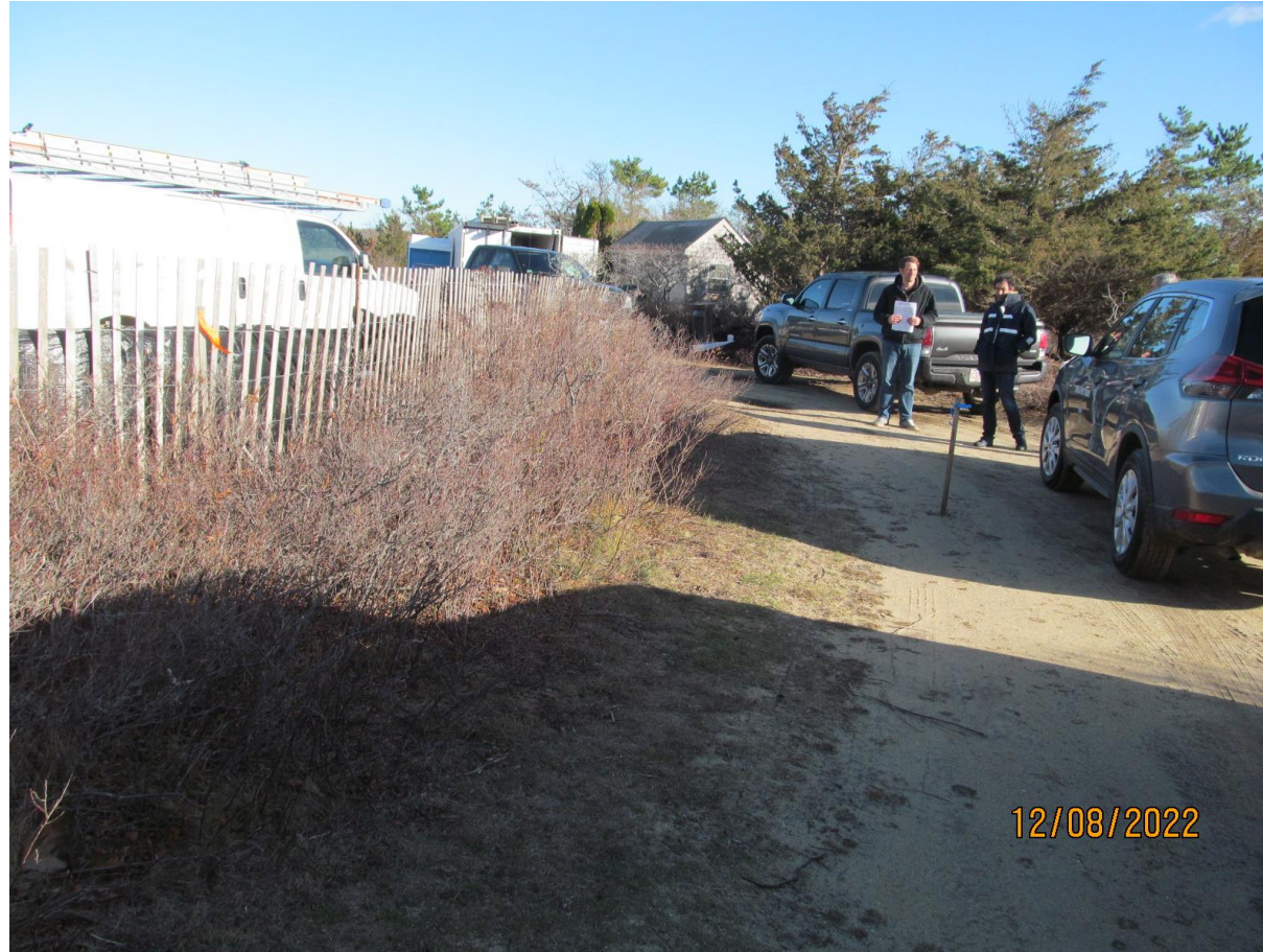
Stake near car is corner of new pool. Outside current limit of work
