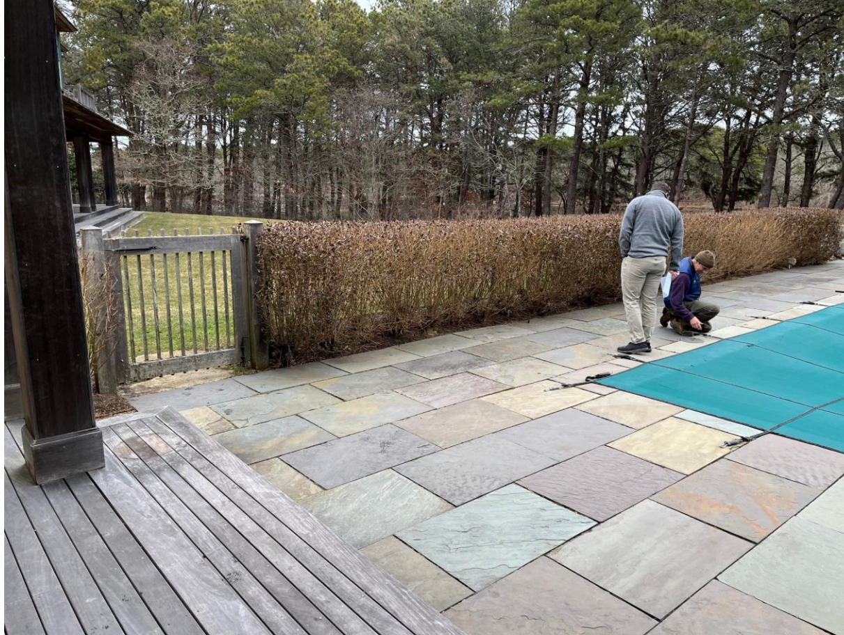
View from deck to the pond. Peter examining the condition of the patio.
