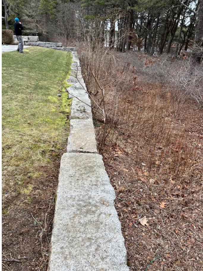
Stone retaining wall along the end of the pool on the pond side.
