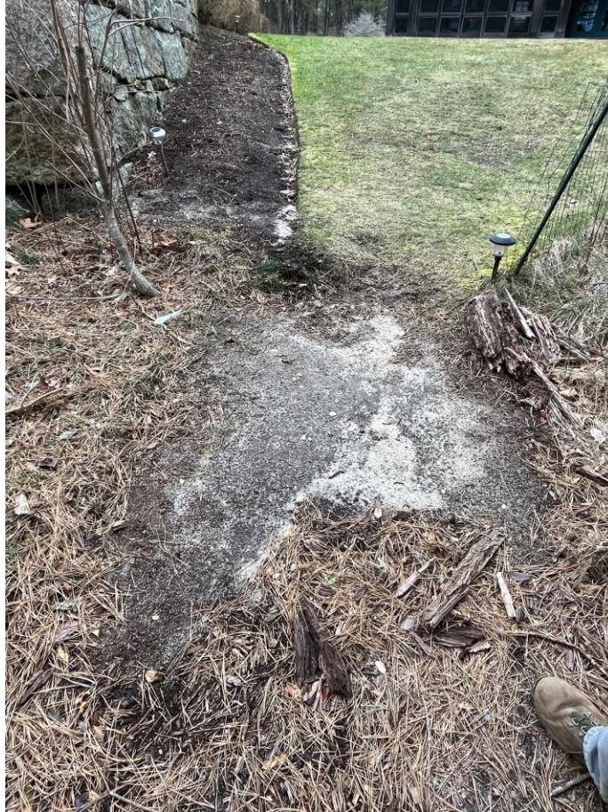
Minor erosion at the end of of the lawn onto the path
