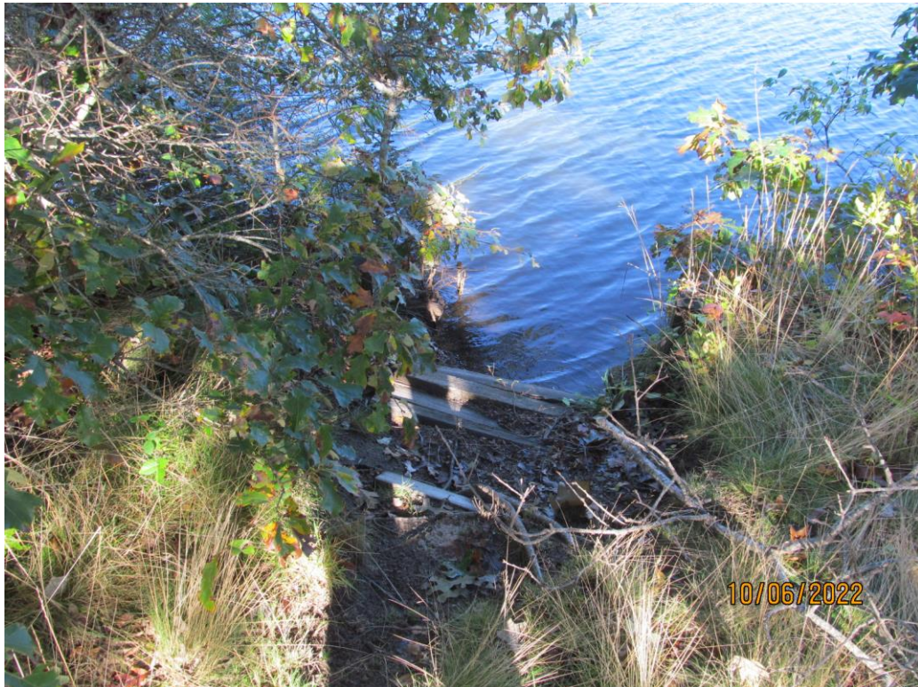
Remanents of old pad for dock
