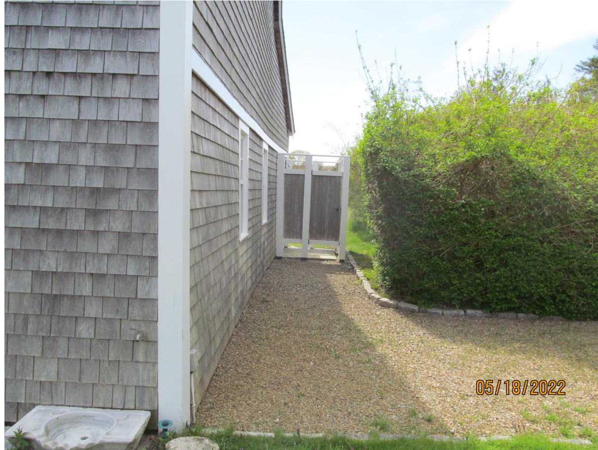
plan called for existing shower to be removed. They must have replaced it.
