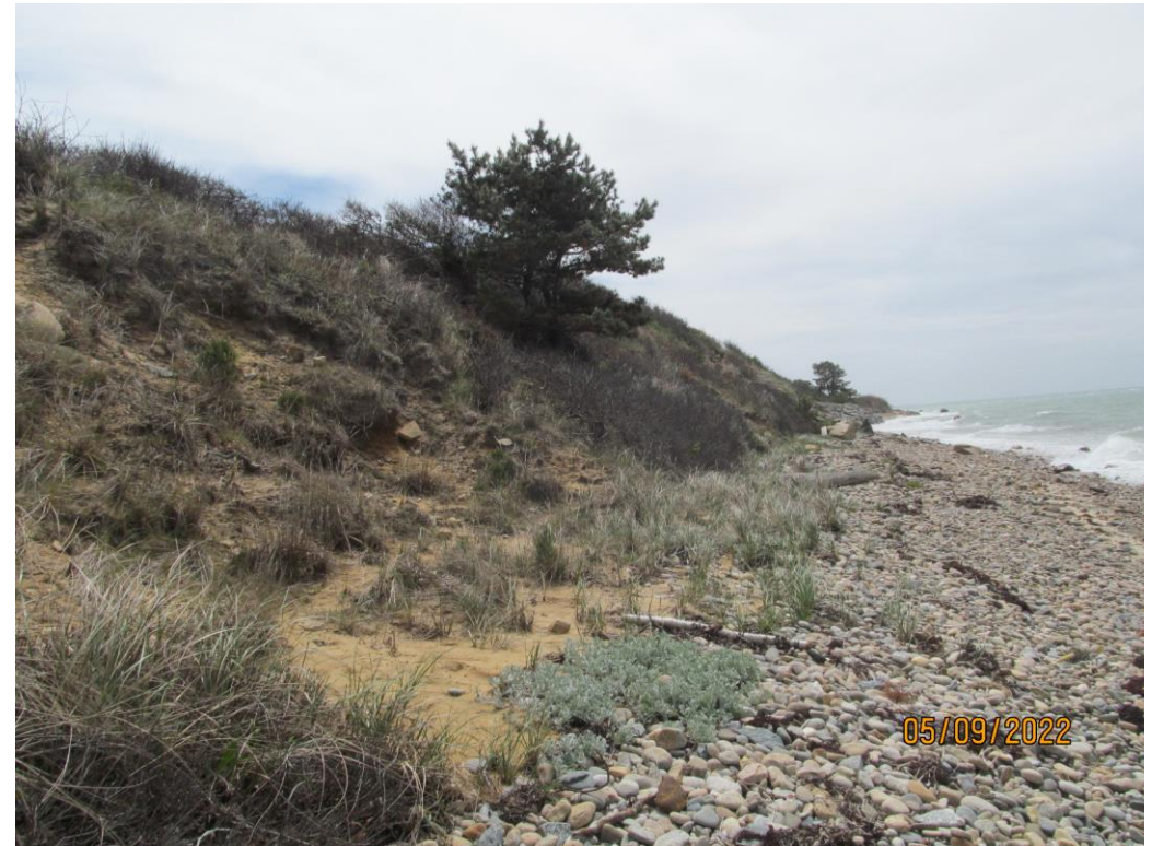
Face of bank looking west. The bank get steeper to the west but is better vegetated.
