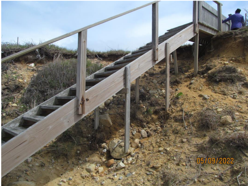
Erosion under stairs. A couple of posts are no longer anchored.
