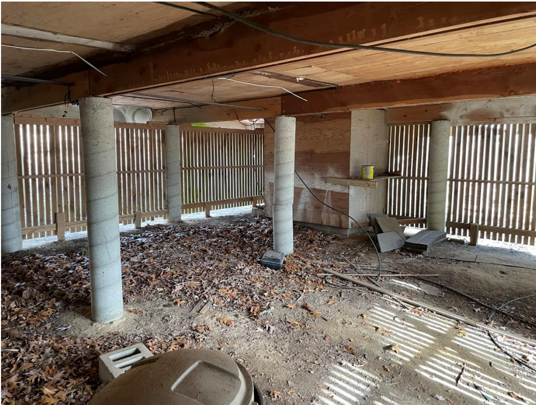
Photograph #4 – View under the existing home that shows the exposed soils and lack of vegetation.
