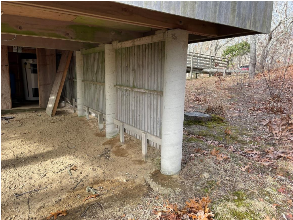
Photograph #6 – View of the piles that support the existing home. Flood waters can travel under the home and be buffered by the Coastal Bank.
