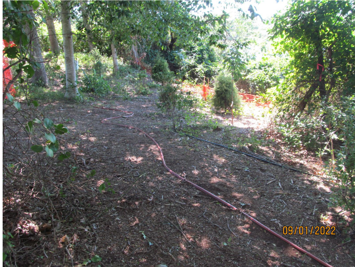
Construction fence is 10ft per plan. Number and speices are in accordance with the plan.
