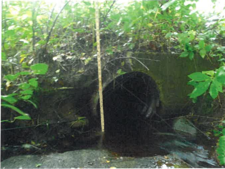
Photo 6: Inlet of culvert at Tiah's Cove Road showing the broken piece of the headwall in the foreground and coaxial cable exiting on the left.
