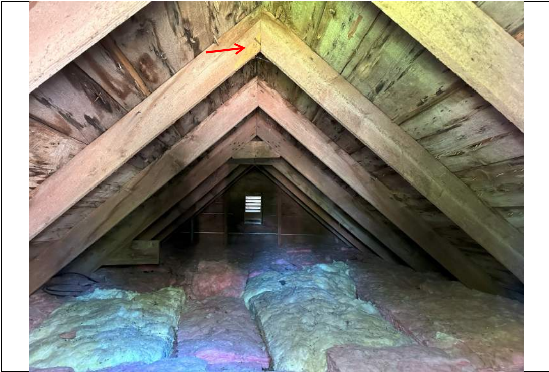
Photograph 4 – View of roof framing looking south. Note deteriorated boards, extensive staining, split at end with exposed corroded nail.
