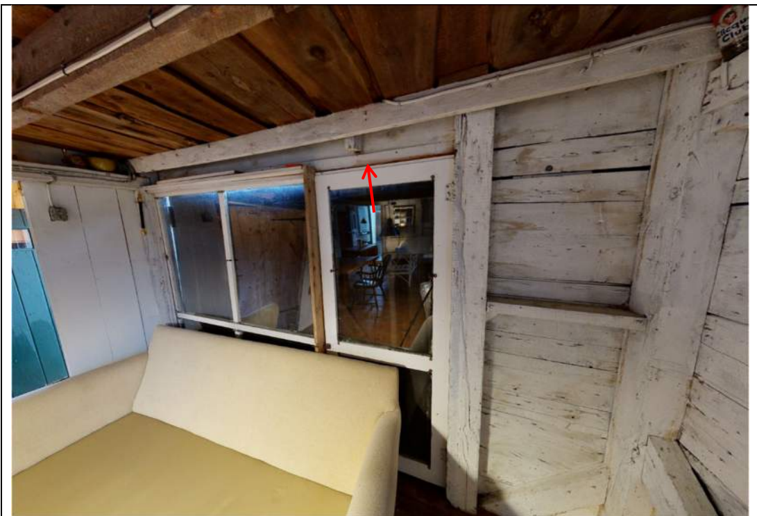
Photograph 10 – View of first floor looking at south door opening. Note lack of header above door.
