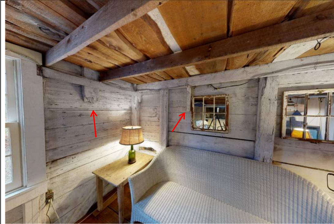
Photograph 9 – View of first floor looking northwest. Note added spacing of posts and 2 nd floor posts that terminate halfway between floors.
