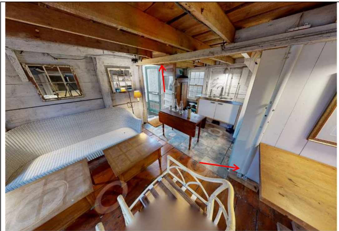
Photograph 8 – View of first floor looking northeast. Note added temporary screw jack column at center beam, and deflection of center beam.
