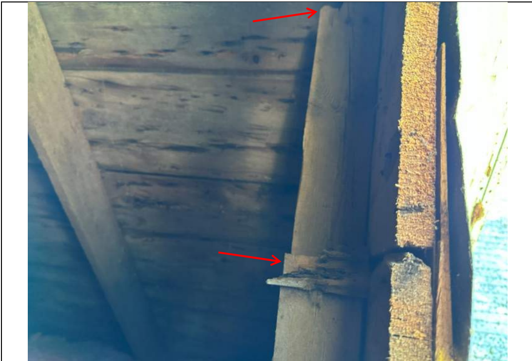
Photograph 6 – View of north gable end wall stud, note deterioration at connections.
