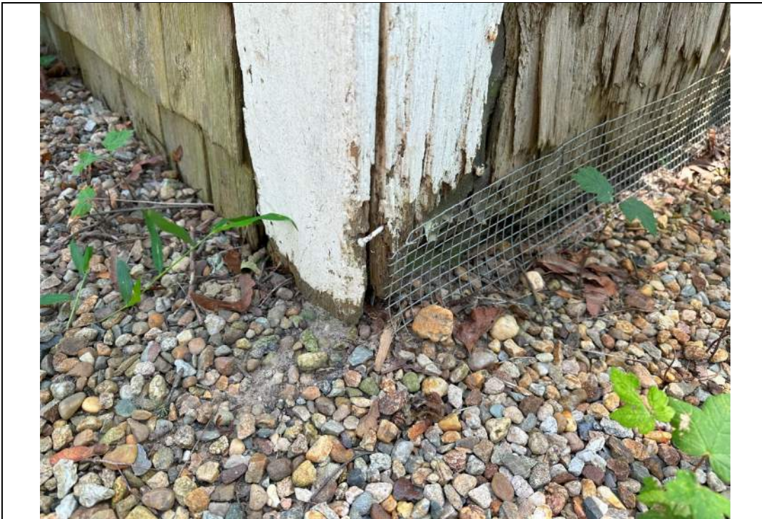
Photograph 2 – Close-up view of Northeast corner. Note deteriorated cladding and horizontal boards beneath
