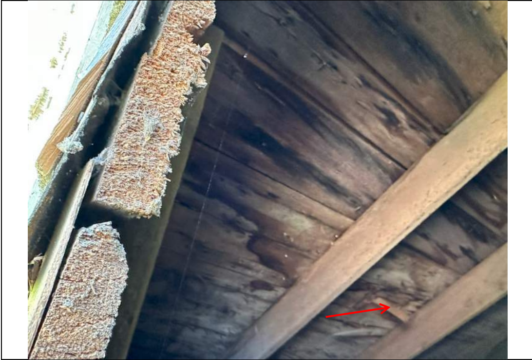
Photograph 5 – Close-up view of north wall boards and deteriorated roof boards (beyond).
