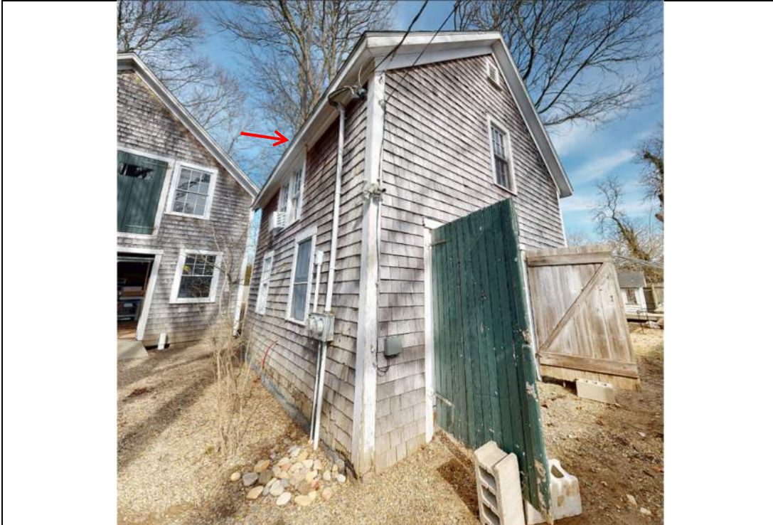
Photograph 1 – View of front (south elevation). Note staining and deteriorated siding at base of walls, and bow in center of roof at the eave
