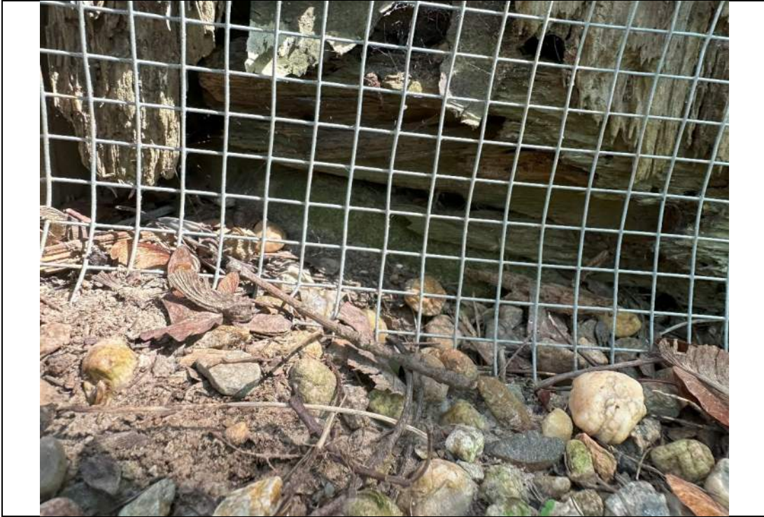
Photograph 3 – Close-up view of deteriorated cladding and bottom plate atop a stone pier.
